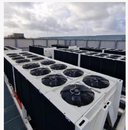
Cooling units fitted with screens
