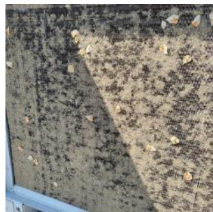
Contamination of condensers
