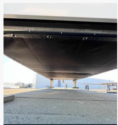
Cooling units equipped with screens
